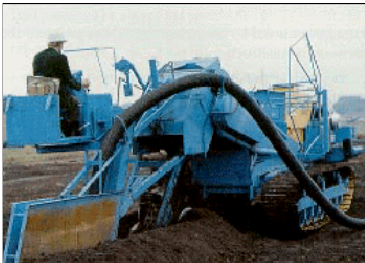
Installing drainage tile. Drainage tile is used extensively in central Illinois to remove excess water from farmland.
